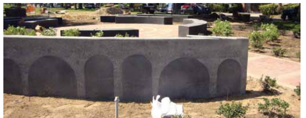
Finishing up the last touches of the Centennial Plaza. Photos by TerriAnn Ferren.
